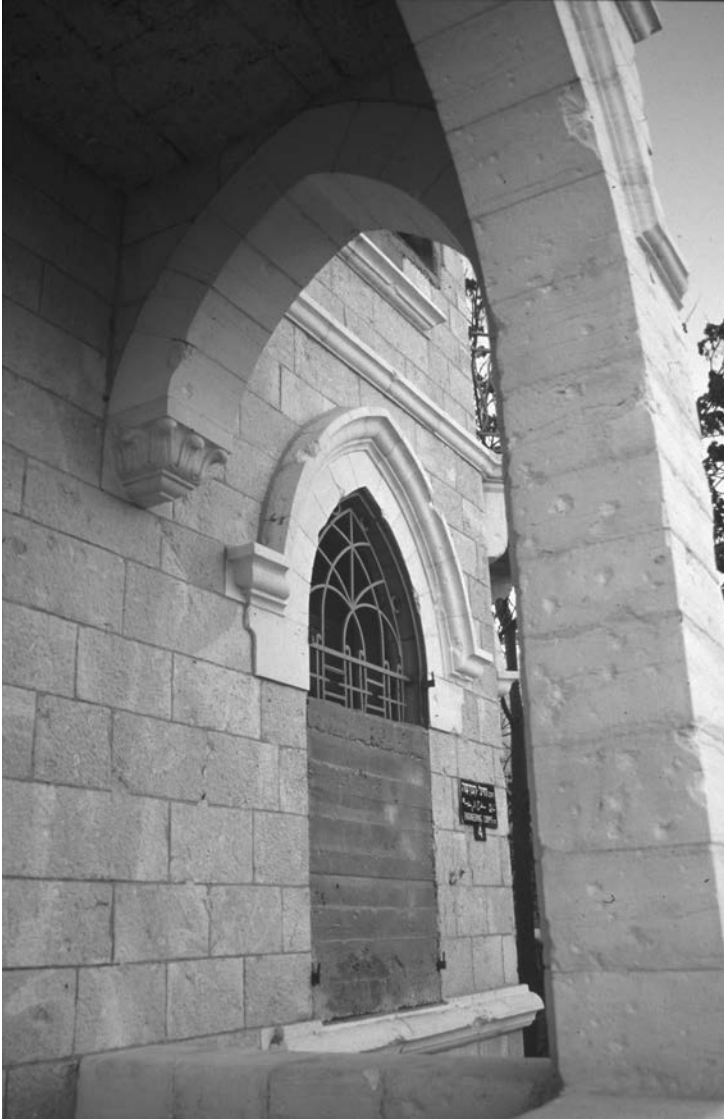
7. The scarred façade of the former Baramki home, 1999. Note the original window filled in with concrete after the Israeli government turned the structure into the Tourjeman Army Post in 1948.
