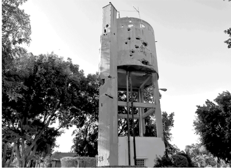
FIGURE 1.4: The old water tower with the bullet holes. Source: Mashka Litvak, a family friend.
