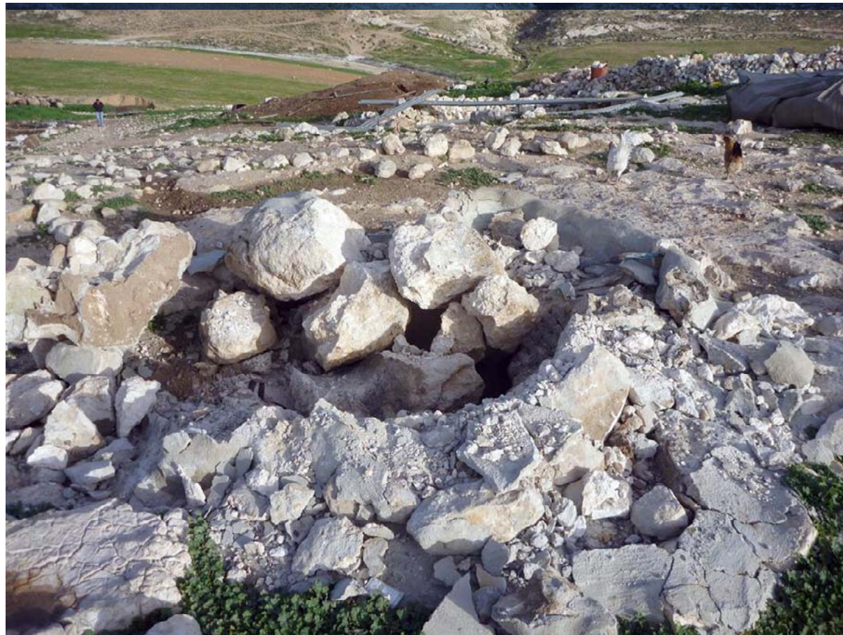
Demolished Polish-funded water cistern in Al-Rihiyya, Hebron governorate – EWASH/PAH©.
