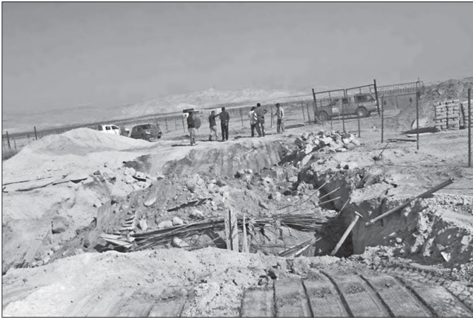
Auja, the West Bank, in Area C: the foundations of the house of Raja Khalidi, the author's brother, bulldozed by the Israeli military
