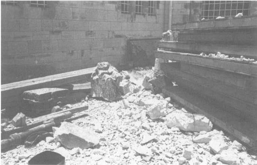
Figure 20. PAM, inner court with damage from the 1967 War. (Photograph by Burger, IAA 49239)
