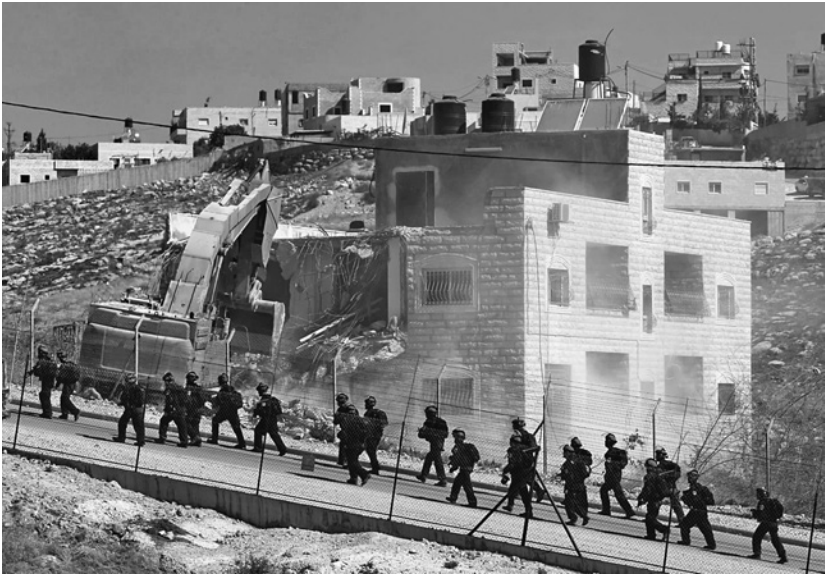
FIGURE 2.6. Israeli security forces accompany the destruction of thirteen buildings, in which seventy families lived, in Sur Baher, East Jerusalem, July 22, 2019. Source: Mussa Issa Qawasma/טרטיוור, in Jecky Huri et al. “The House Demolition in East Jerusalem Is a Ruthless Attack on Simple People,” Ha’aretz , July 22, 2019, https://www.haaretz.co.il/news/politics/.premium-1.7547975 .
