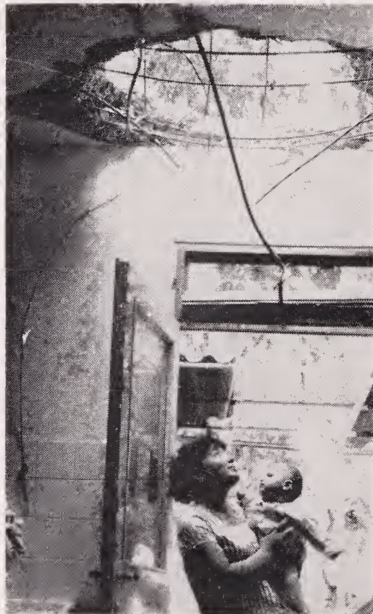
FIG. 16. Examining the damage after the shelling of the crèche in a "border incident". The children of this kibbutz had been taken to the shelters before the attack. (Moshe Lapidot [Mizra].)
