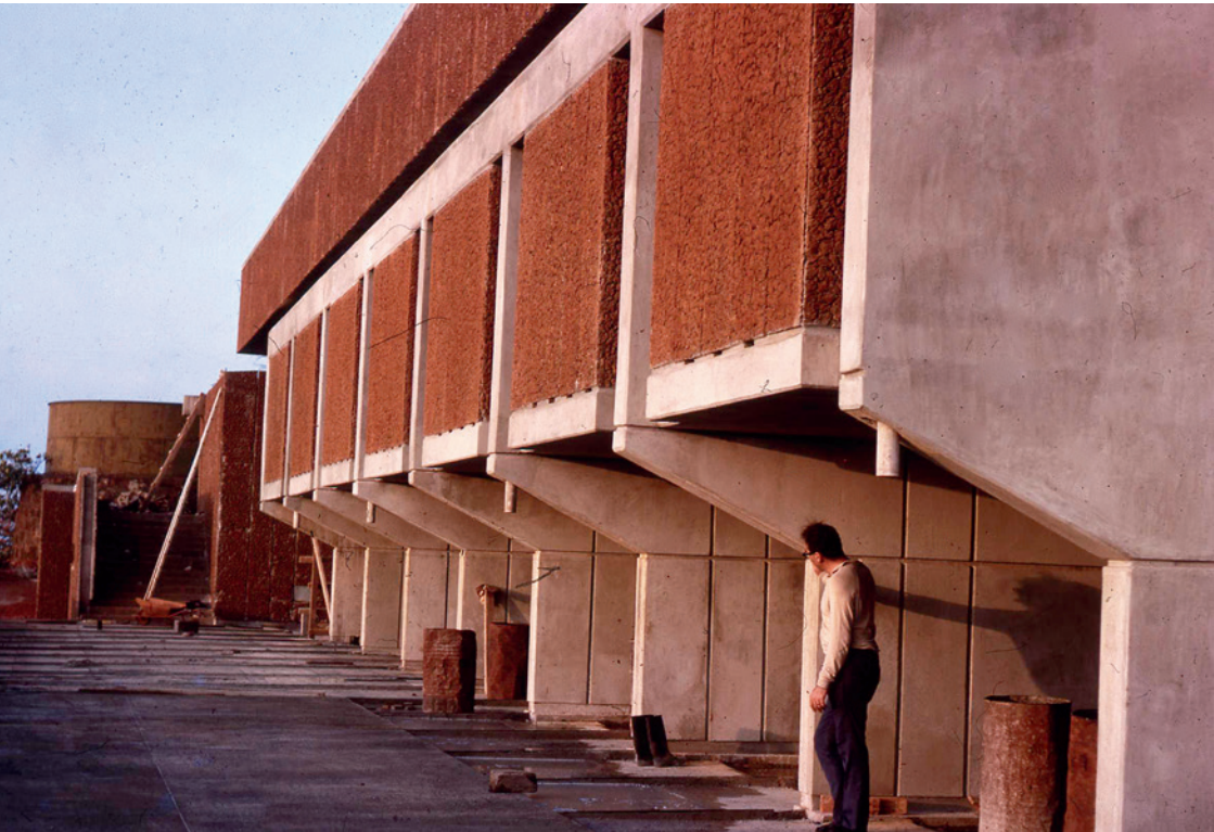
PLATE 2 (TOP) Sierra Leone parliament southern facade, Freetown, 1960. Courtesy of the Azrieli Architectural Archive; Dov and Ram Karmi collection, 8267357058013. PLATE 3 (BOTTOM) Sierra Leone parliament western facade, Freetown, 1960. Courtesy of the Azrieli Architectural Archive; Dov and Ram Karmi collection, 8267357058013.
