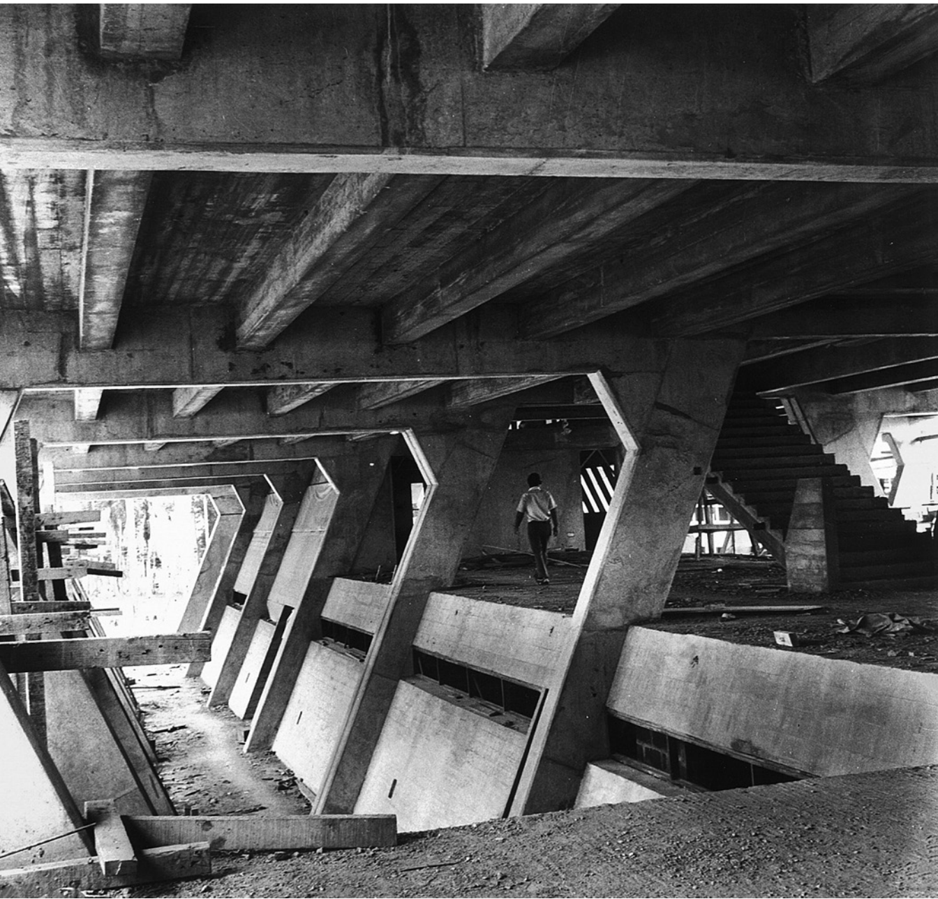
FIGURE 4.14 Faculty of Education under construction, University of Ife, early 1970s. Courtesy of Amos Spitz.
