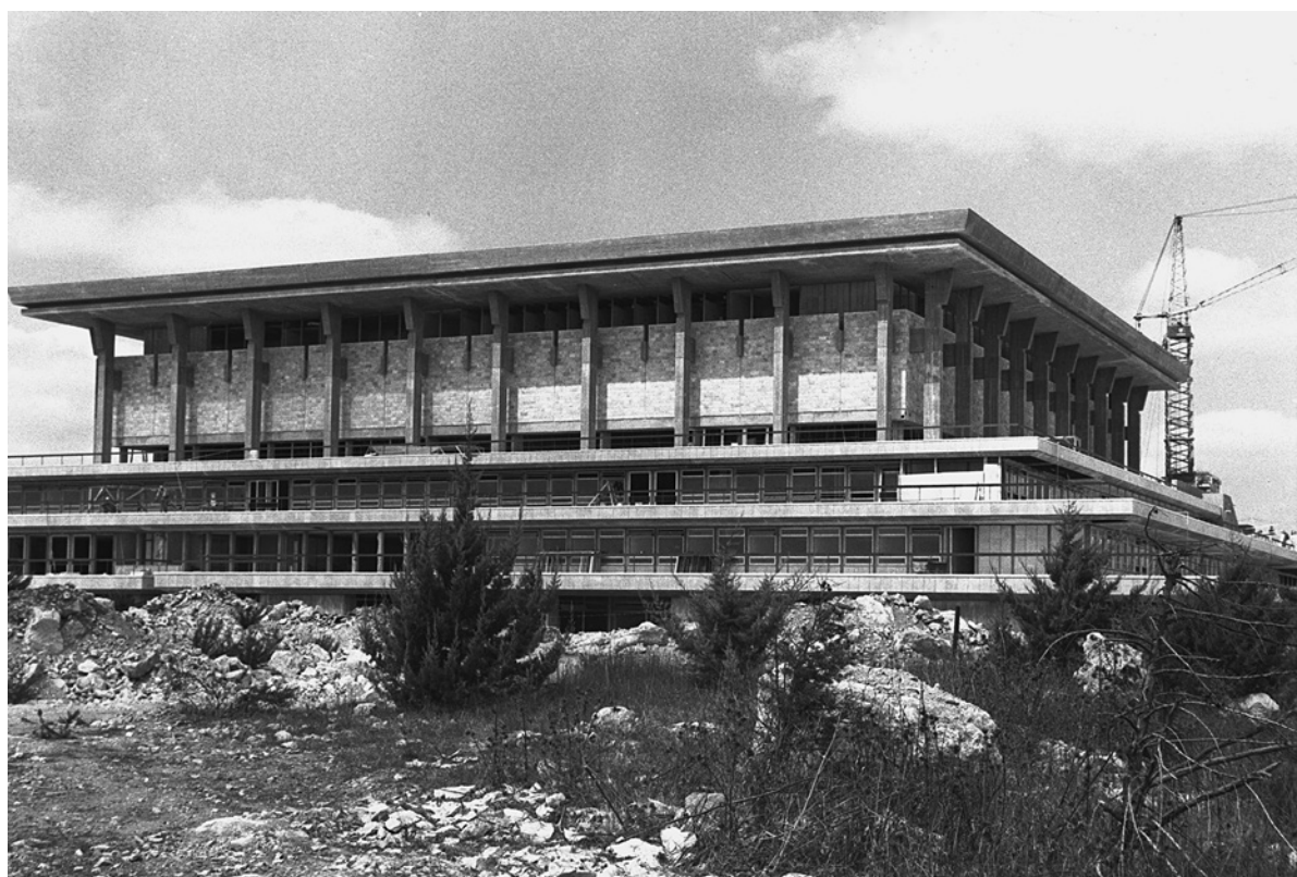
FIGURE 1.4 The Knesset under construction, Jerusalem, early 1960s. Photograph: Moshe Fridan, Israel Government Press Archive.
