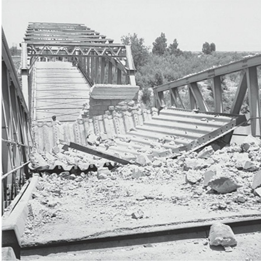
Damage to the Allenby Bridge carrying the main road from Palestine to Transjordan following an attack by underground saboteurs, June 1946. (Photo Sergeant Gregory)
