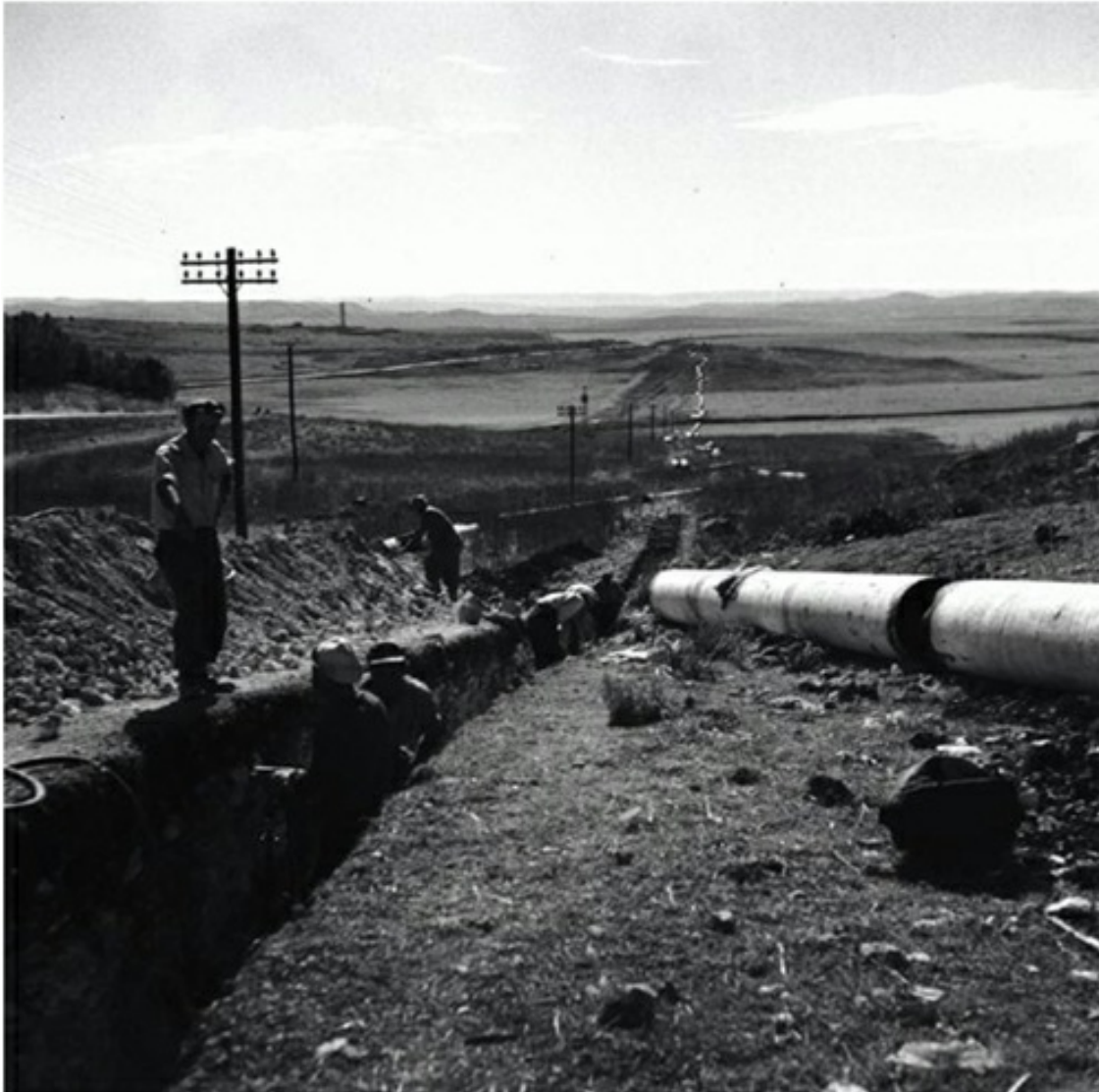
Figure 4.1 Piping water from the Nahr al Auja to Jerusalem towards the end of the Mandate. Laying water pipe to Jerusalem, c. 1946 Werner Braun - kkl-jnf photo archive via the PikiWiki - Israel free image collection project https://en.wikipedia.org/wiki/Water_supply_and_sanitation_in_Israel#/media/File:PikiWiki_Israel_14794_water_to_Jerusalem.jp
